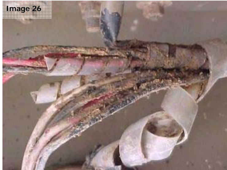
Image 26: All looming around hydraulic and electrical cables is to be verified free of contamination.
