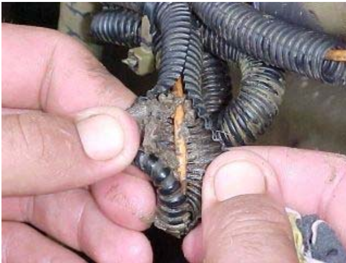
Image 27: All wiring harnesses are to be cleaned and checked for any contamination.
